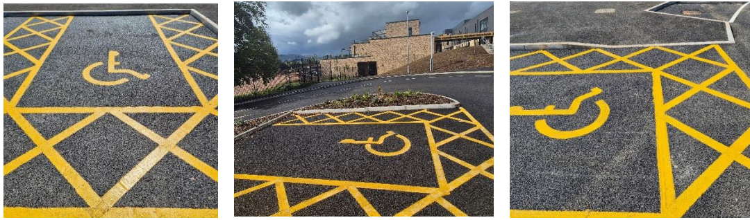
Disabled parking bays adjacent to the Main School Entrance and Lower Phase School Building
